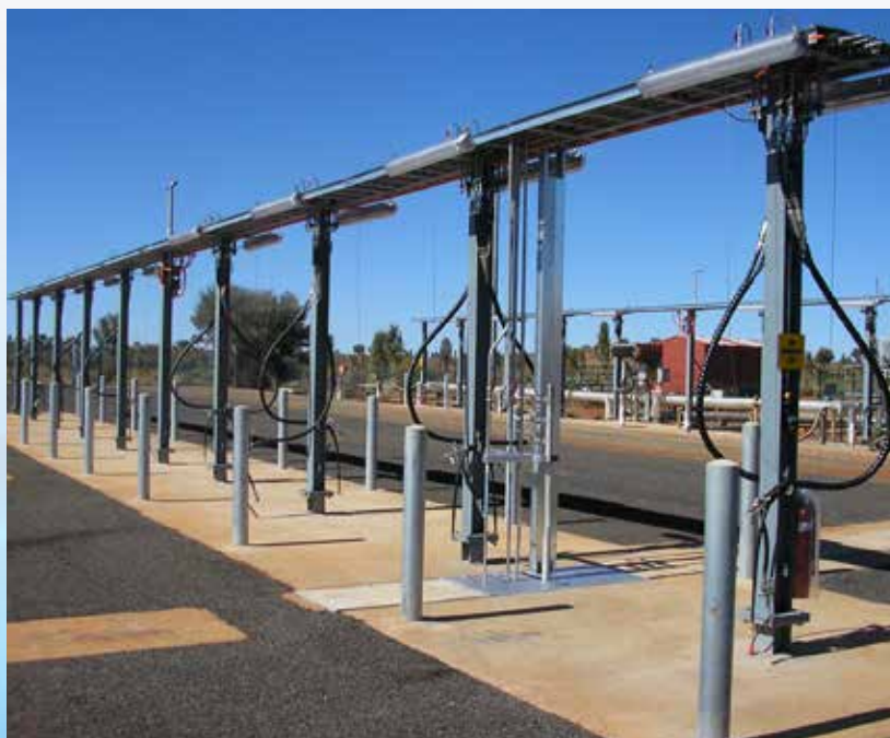
CNG Unloading Facility at Yulara
