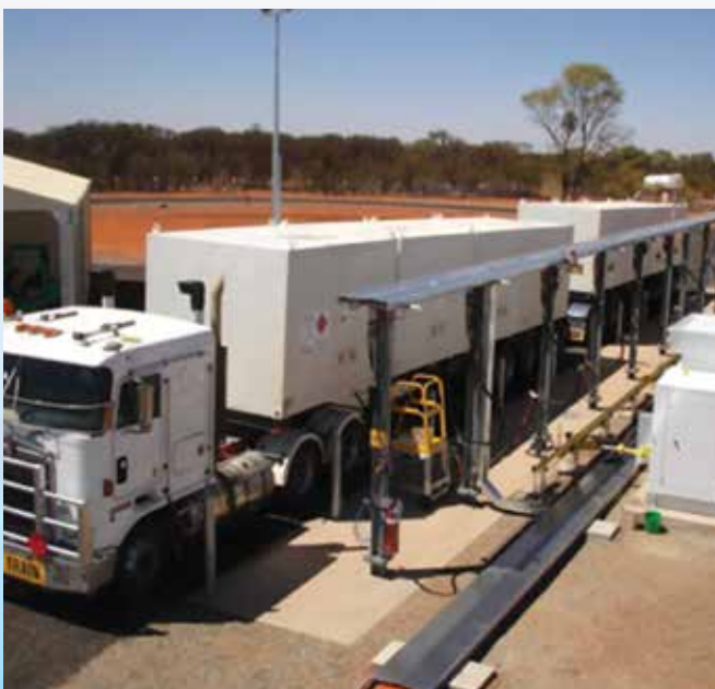
Alice Springs CNG Compression Facility
